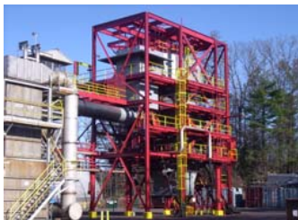
Alstom BSF Windsor US - 15 MWth
