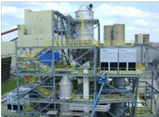
AEP Mountaineer USA - 58 MWth
