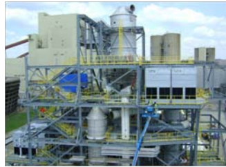
AEP Mountaineer USA - 58 MWth Chilled Ammonia - Coal
