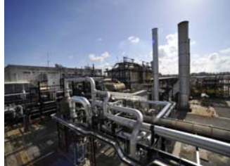
Total Lacq France - 30 MWth Oxy - Gas
