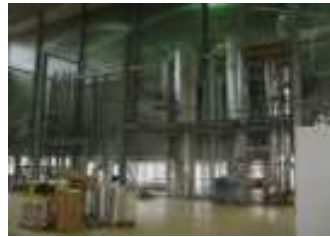
EoN Karlshamn Sweden - 5 MWth
