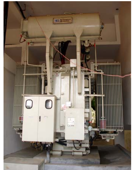
Residential substation transformer
