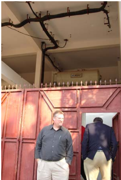
Security gate at residential substation
