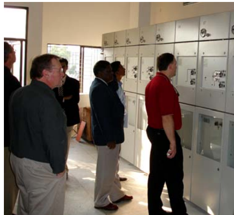
Clark Public Utilities delegation inspects new control panel at DESCO' newest Substation
