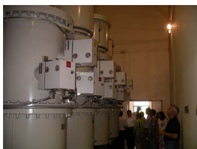
TEIAS 400 kv Substation (top) and Enclosed Substation Gas Busbar (bottom)
