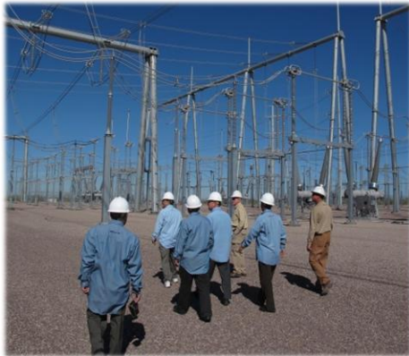
NEPCO and APS delegates inspect GE and Hyundai transformers at APS's Pinnacle Peak substation. APS is currently in the process of expanding this substation in order to prepare for electricity generated by renewable energy projects under construction.
