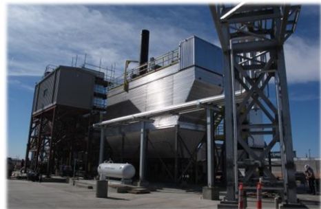
PepsiCo's new biomass boiler at their Frito Lay facility in Casa Grande, AZ. This combined heat and power plant will provide steam and electricity to manufacturing operations and displace 80% of the facilities natural gas needs.
