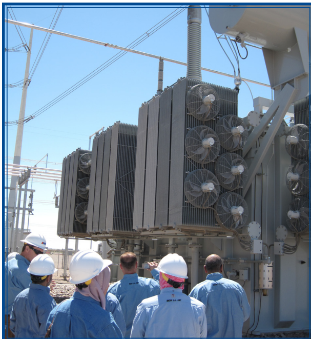
NEPCO delegates inspect a high-voltage transformer at a 500-345 kV APS substation.
