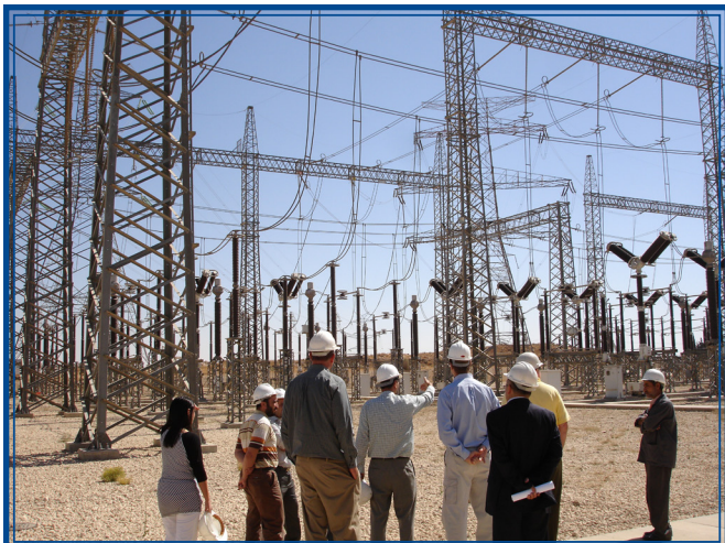
APS executives visit NEPCO's Amman South substation.
