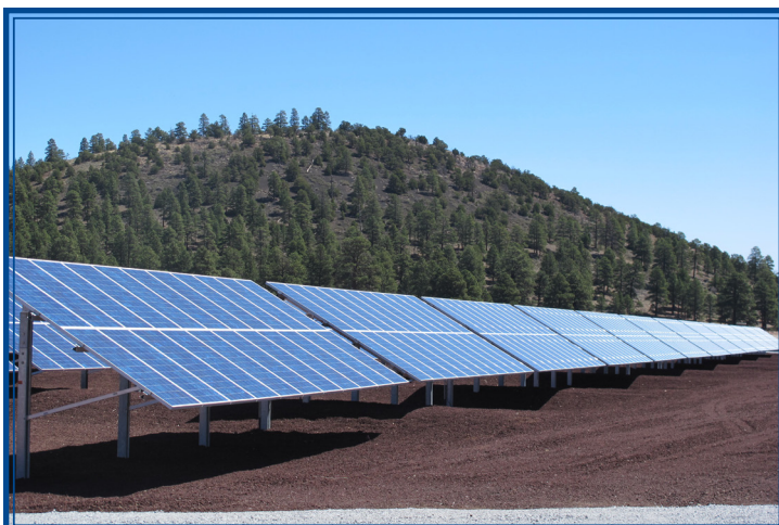
APS’s Doney Park Renewable Energy Site near Flagstaff, AZ.
