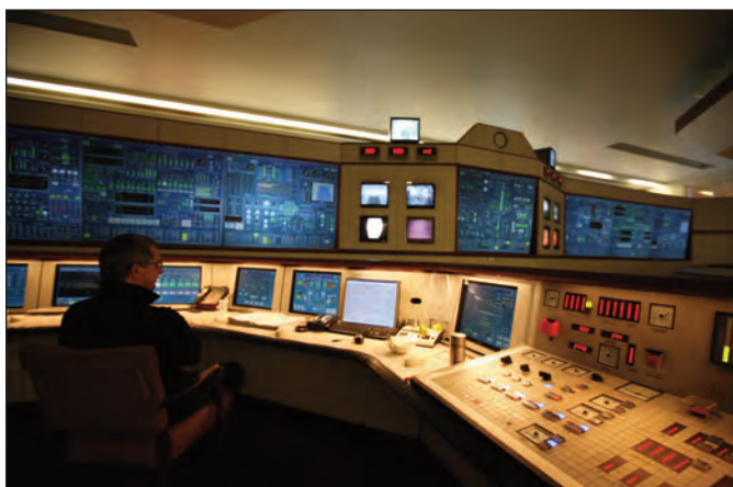
Figure 17 Updated plant control system installed in International Power's 2 GW Rugeley B station (photograph courtesy of Russell Mills Photography)
