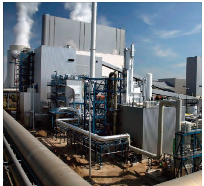
Figure 7 The oxyfuel boiler assembly of the Schwarze Pumpe pilot plant in Germany (photograph courtesy of Vattenfall)
