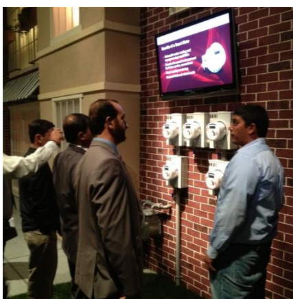
Above: The PDP delegation visits Duke Energy's Envision Center, which gives an interactive tour of Duke's cutting-edge research in energy efficiency for residential consumers. Here, examples of state-of-the-art smart meters are displayed.
